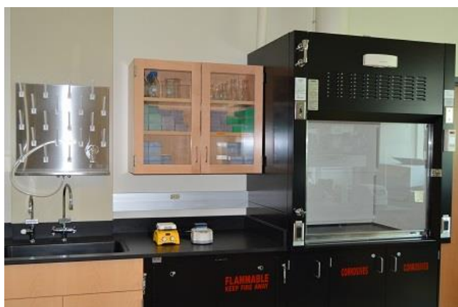
Mott fume hood next to sink.
